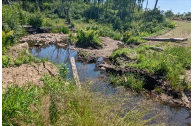
Uninstalled culverts sit beside damaged creek (road VMR-1B-1B).
