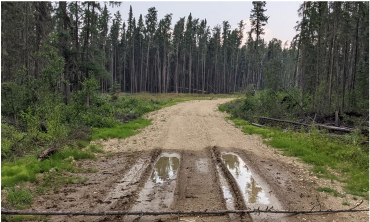
Water sitting on road in improper wetland crossing (road LNK-1A).
