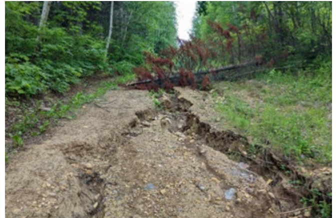
Washed out logging road (road CWC-5-1).
