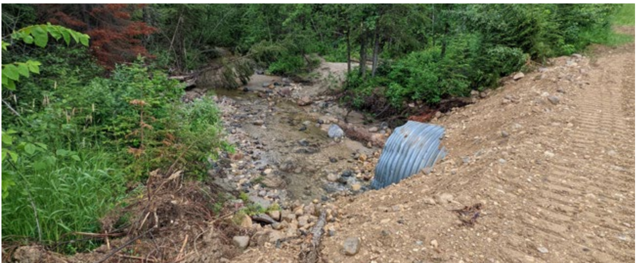
Replacement culvert and downstream sedimentation (Vimy Ridge Road).
