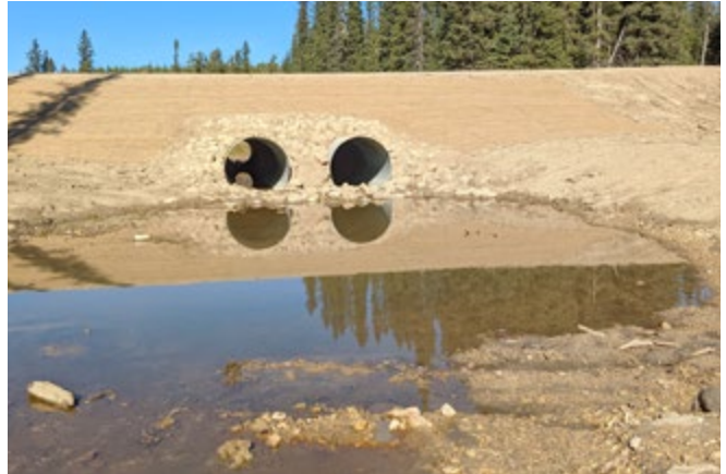
New inadequately sized culverts on Highway 367.
