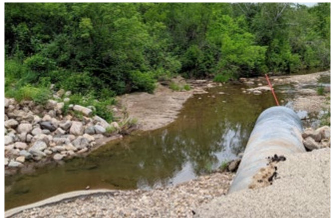
Washout on Highway 367.
