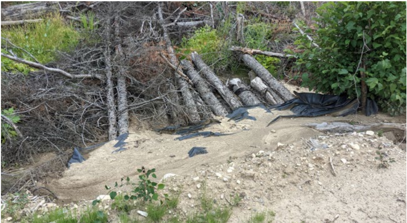
Road over wetland without culvert and with sediment polluting wetland (road LNK-1B).
