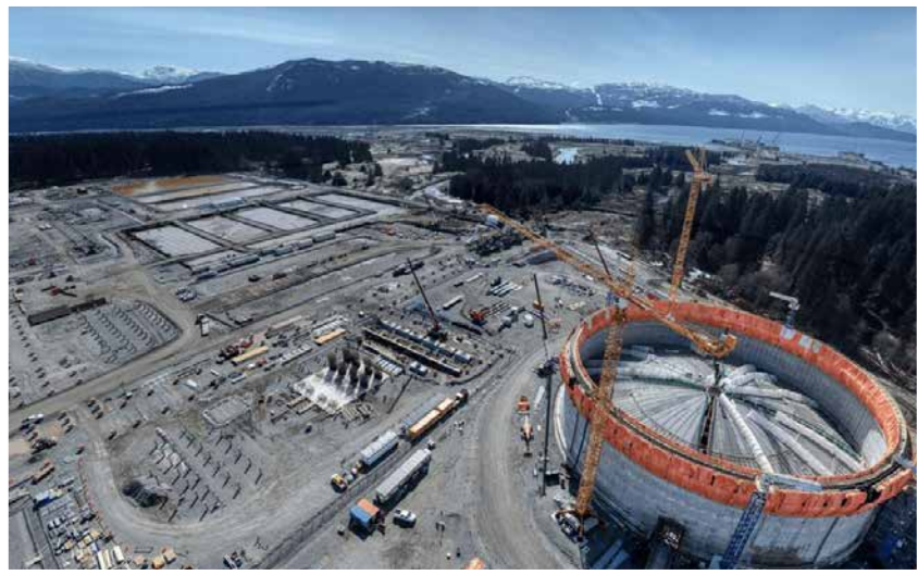
Photo: LNG Canada phase one is under construction in Kitimat, B.C. (WC files).
