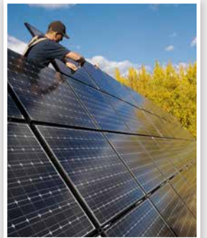
Photo: Worker installing a solar panel at the Riverdale Net-Zero Project in Edmonton, AB (Gordon Howell).
