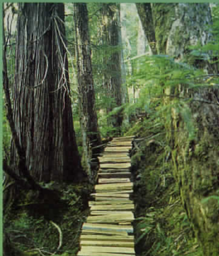
Thick, hand-split cedar treads cover "Witness Trail" boardwalk built by WCWC volunteers in 1993-94.
